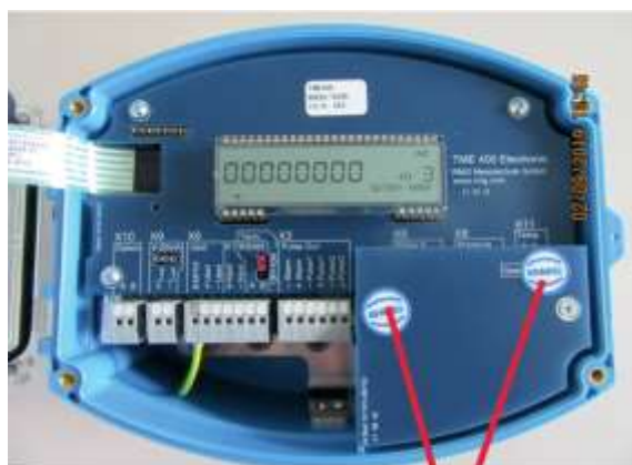
In the electronic enclosure
