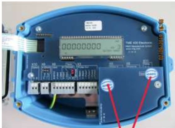
In the electronic enclosure
